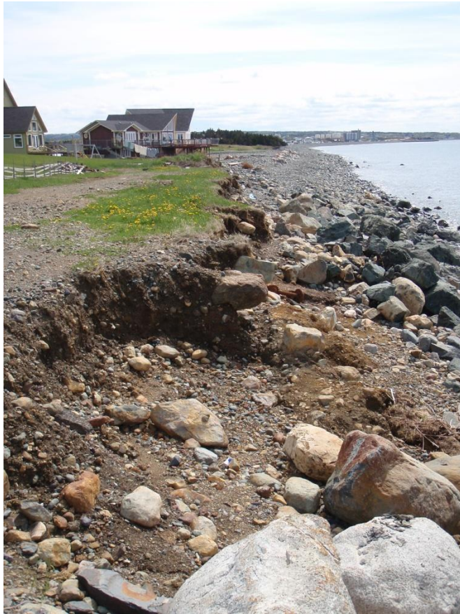
Figure 4: Damaged shoreline near Cherry Lane (Source: Personal Photo)
