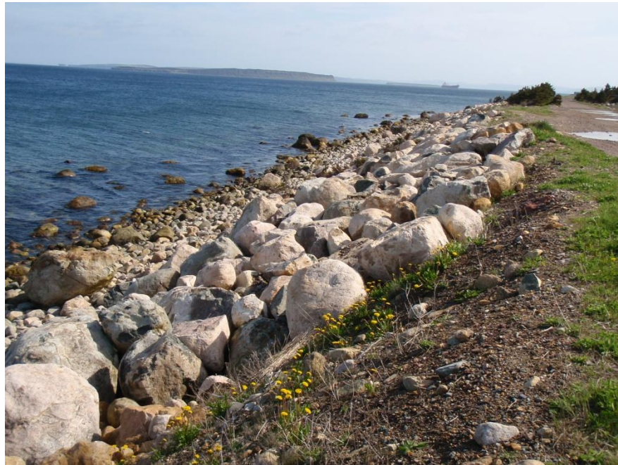
Figure 3: Revetment located near Anthony's Road (Source: Personal Photo)
