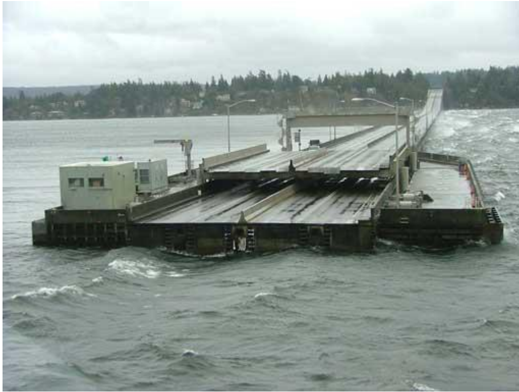
Figure 2: Retracted drawspan on the SR 520 Bridge to relieve pressure during a storm
