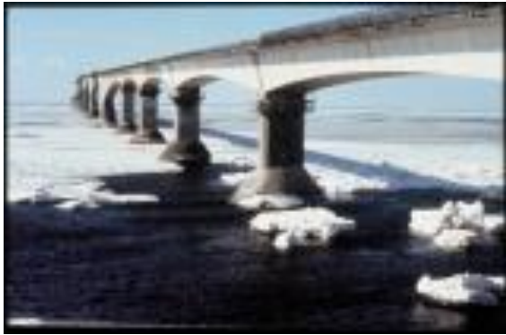
Figure 4: Confederation Bridge as it is subject to ice floes and ice loading [9]
