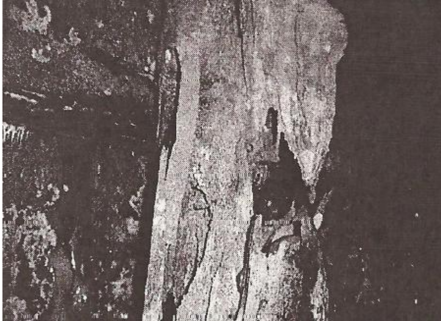
Figure 4: A creosote treated timber pile which is approximately 90% deteriorated due to rot [2].
