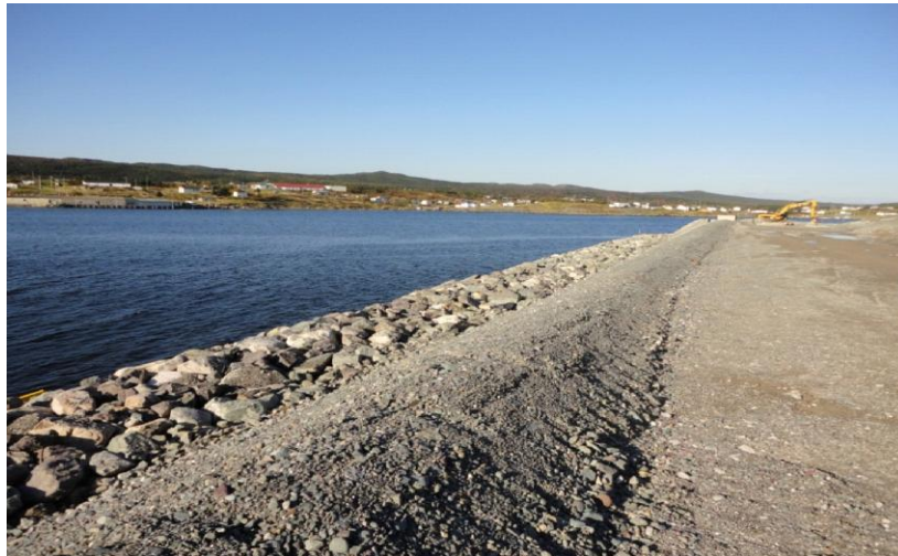
Figure 4: Shoreline Protection. Photo credited to PMJV.
