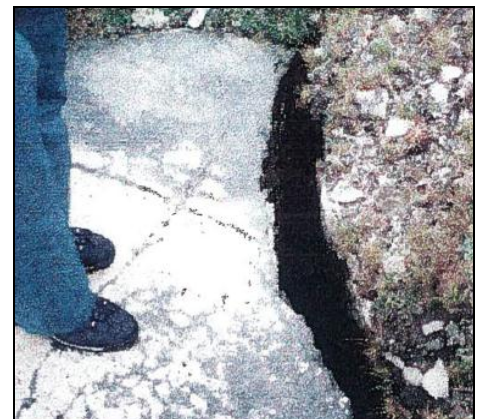
Figure 5: Tension Crack 1 to 3 m From Cliff [5]
